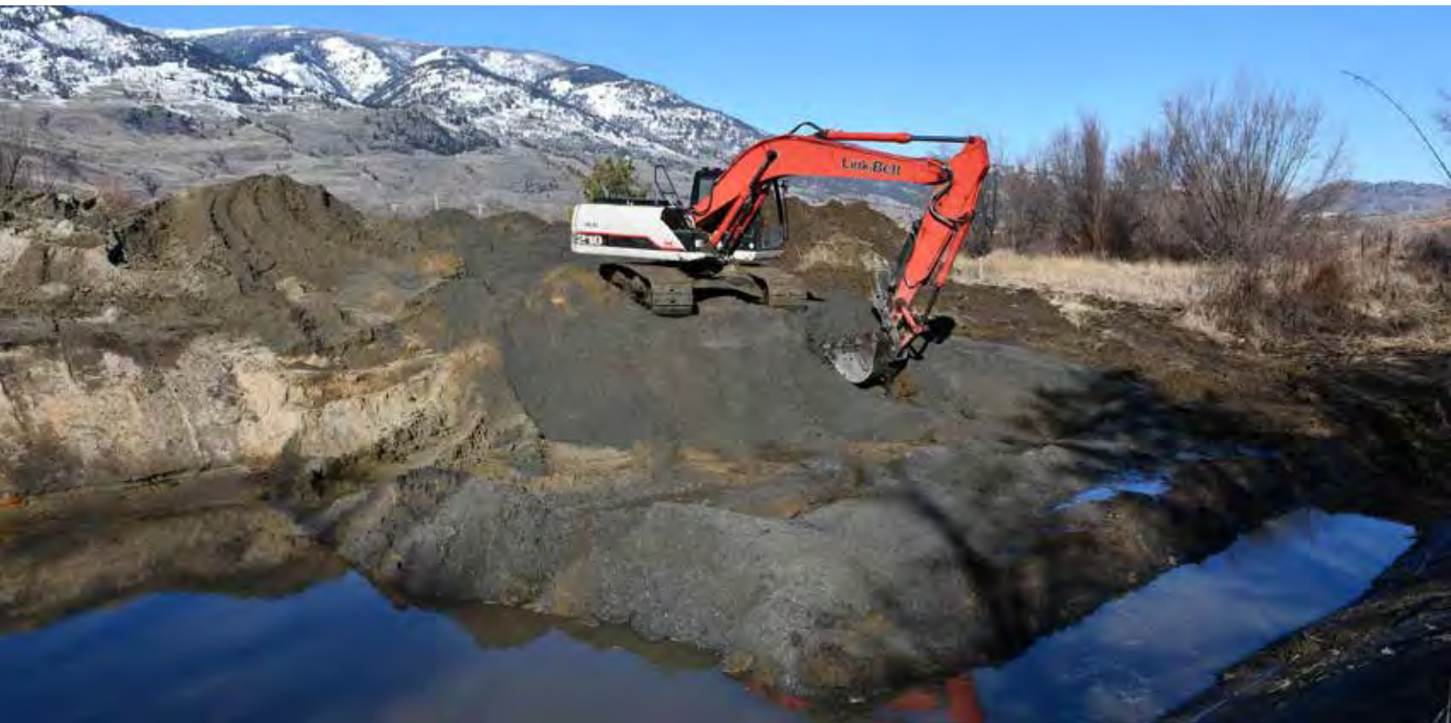
Wetland construction underway on the Winters property, southern British Columbia. Ducks Unlimited Canada
