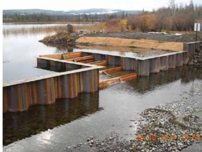
The newly built weir and fishway stabilizes water levels in Fletcher Lake for the benefit of waterfowl and other birds. Ducks Unlimited Canada
