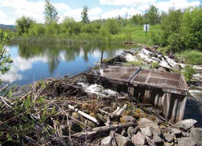
The original weir built in 1980 at Fletcher Lake, BC. Ducks Unlimited Canada
